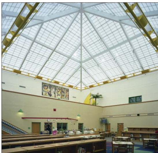
The pyramid skylight in an Elkhart, Indiana, elementary school uses Kalwall composite glazing with insulating Nanogel silica aerogel. Nanogel has been certified for low manufacturing impacts in Cradle to Cradle and evaluated for its performance through the GreenSpec Directory. Photo: Bill Lempke
